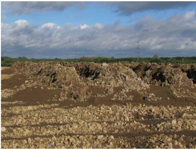
Figure 3. Dumping of the sludge in ridges during the construction of test embankment to enhance drying by wind and sun
