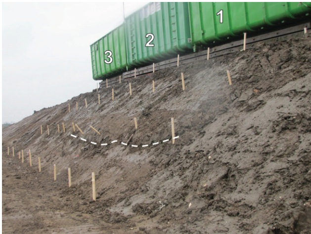
Figure 10. Bulge formed below container 1, just above the interface between the sand layer and the sludge
