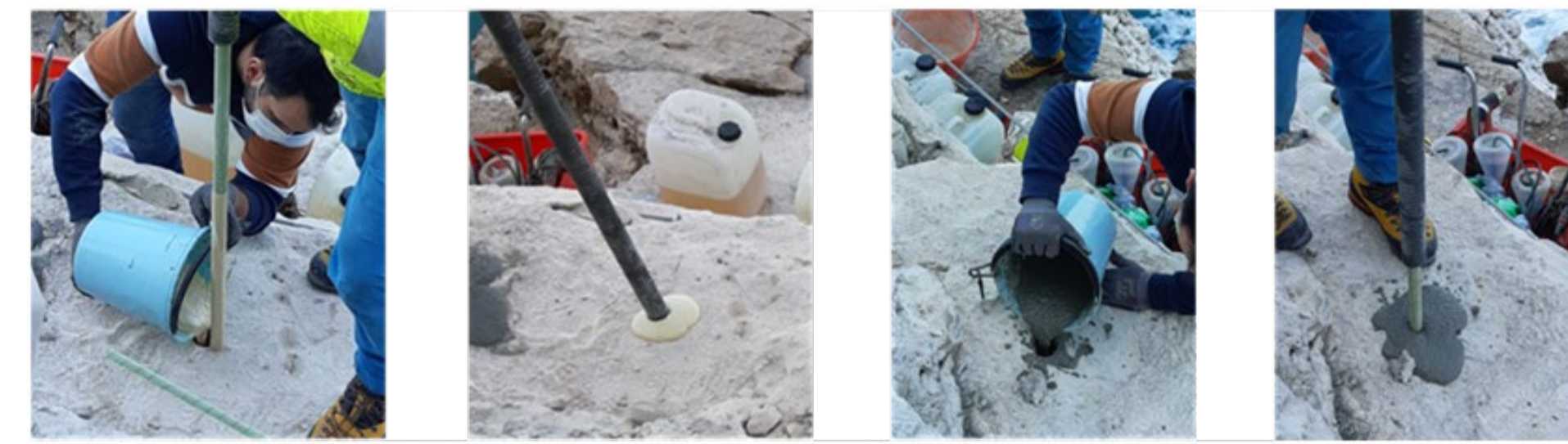
Figure 3 pouring to two different materials (MasterEmaco T 1200 PG and MasterRoc RBA 380) in CB
