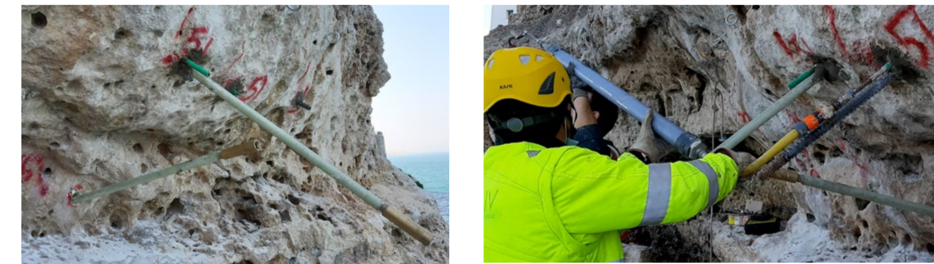
Figure 2 a) GFRP bars blocked by Lampocem before injection; b) injection of MasterEmaco 222 through injection tube in CG
