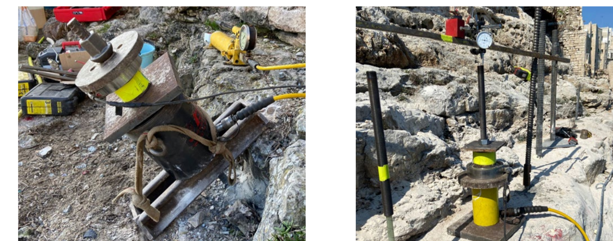
Figure 4 a) Pull test with 1000 kN capacity Hallow piston; b) pull test with 300 kN capacity hallow piston
