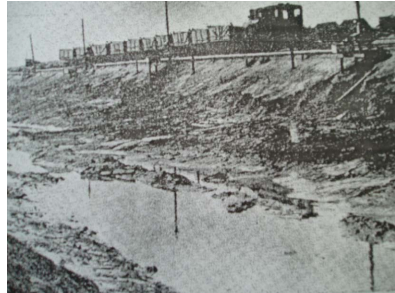
EO Treatment 7m deep steel electrodes @ 9m and 180V Work recommenced after 2 days, 1.3 kWhr/m 3 of excavation
