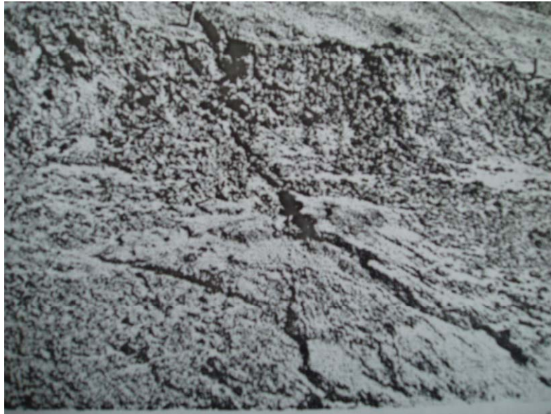
Clay/silt cutting Work stopped due to instability
